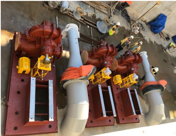
Internal components of Water Treatment Plant
