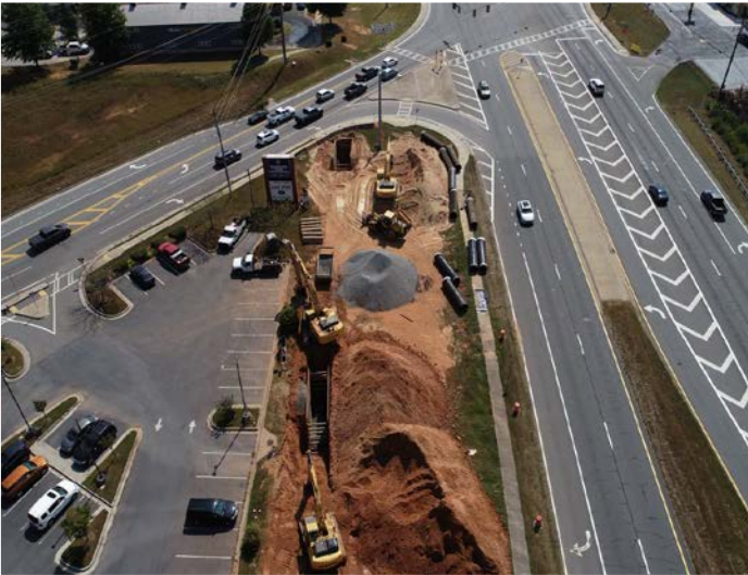
Pipeline path at the intersection of Mars Hill Road and U.S. Highway 41 in Acworth, GA
