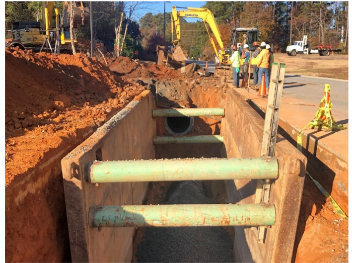
New pipeline being installed in the same trench location as the old pipeline
