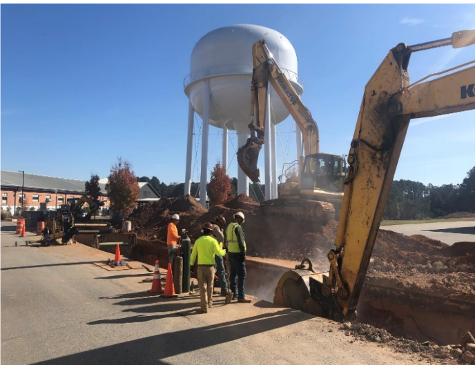
Construction progress at Wyckoff Water Treatment Plant, leading to connection of new pipeline to the treatment plant
