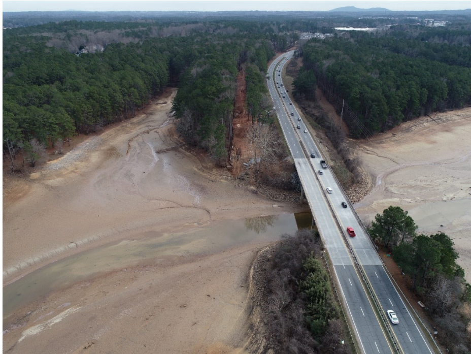
Pipeline path will run parallel to U.S. Highway 41 and will cross under Allatoona Lake. This project was planned to reach this location in the winter when lake levels are low enough to allow for construction.
