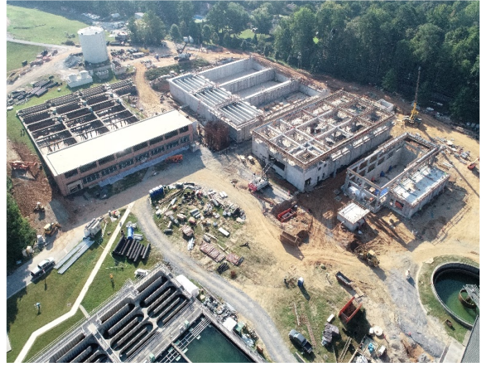
Aerial view of construction progress before the old Quarles Plant 1 (on left) was completely demolished
