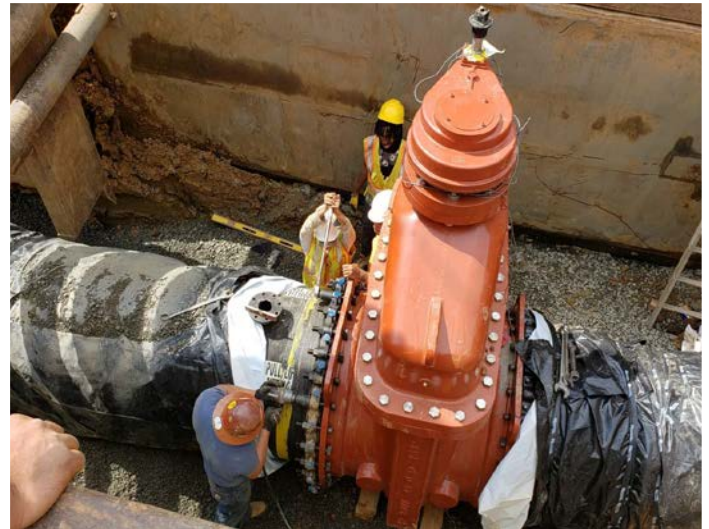
36" gate valve outside the Wyckoff Water Treatment Plant, which allows operators to control flows leaving the treatment plant
