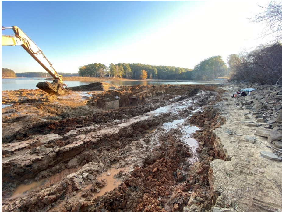
Pipeline path runs parallel to U.S. Highway 41 and crosses under Allatoona Lake. The lake crossing was planned for winter when lake levels are low enough to allow for construction. This picture shows the pipeline path in an area usually covered by water.
