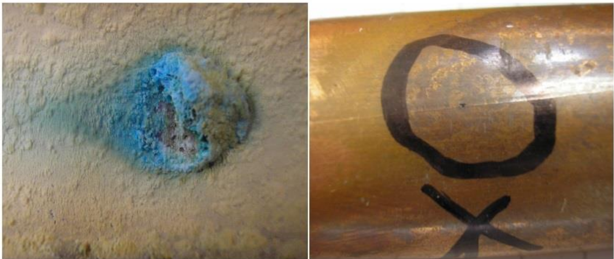
Figure 3: (specimen Z) Photo on left shows a typical water-side pitting site with characteristic blue green tuberculation. Photo on right shows the pinhole sized point of penetration on the exterior of the pipe opposite the pit.
