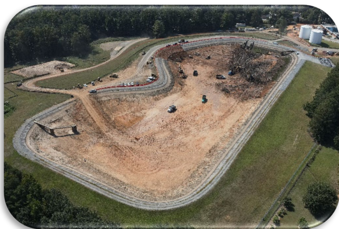
Quarles Water Treatment Plant Reservoir Empty for Cleaning
